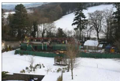
The roof beams were positioned ready for the joiners to work on the beams.
