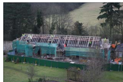
The shape of the building becomes apparent once the roof beams are fixed by the joiners.
