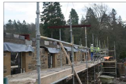
By January 2009 the build was up to the first floor and steel supports were manoeuvred into place.
