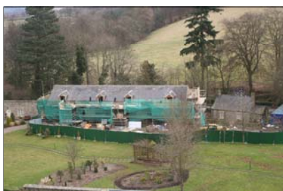
With the roof tiles on, the building is almost water-tight and work inside the building can continue.
